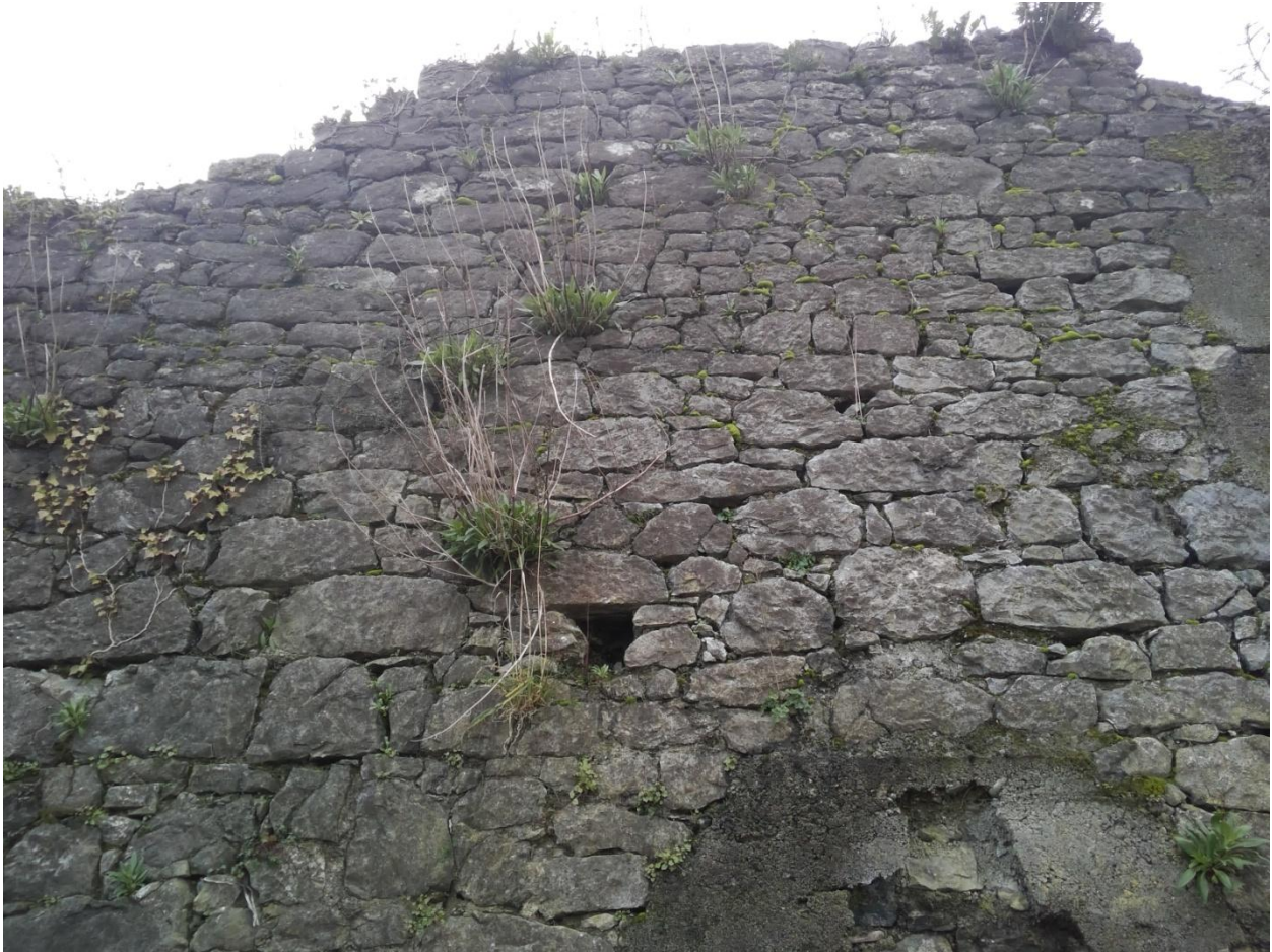
Pic 3: Detail of south part of subject wall (close to Burke Street). The haunching at the top of the wall has broken down with colonisation by buddleia and ivy. There are loose and unstable stones along the top of the wall.
