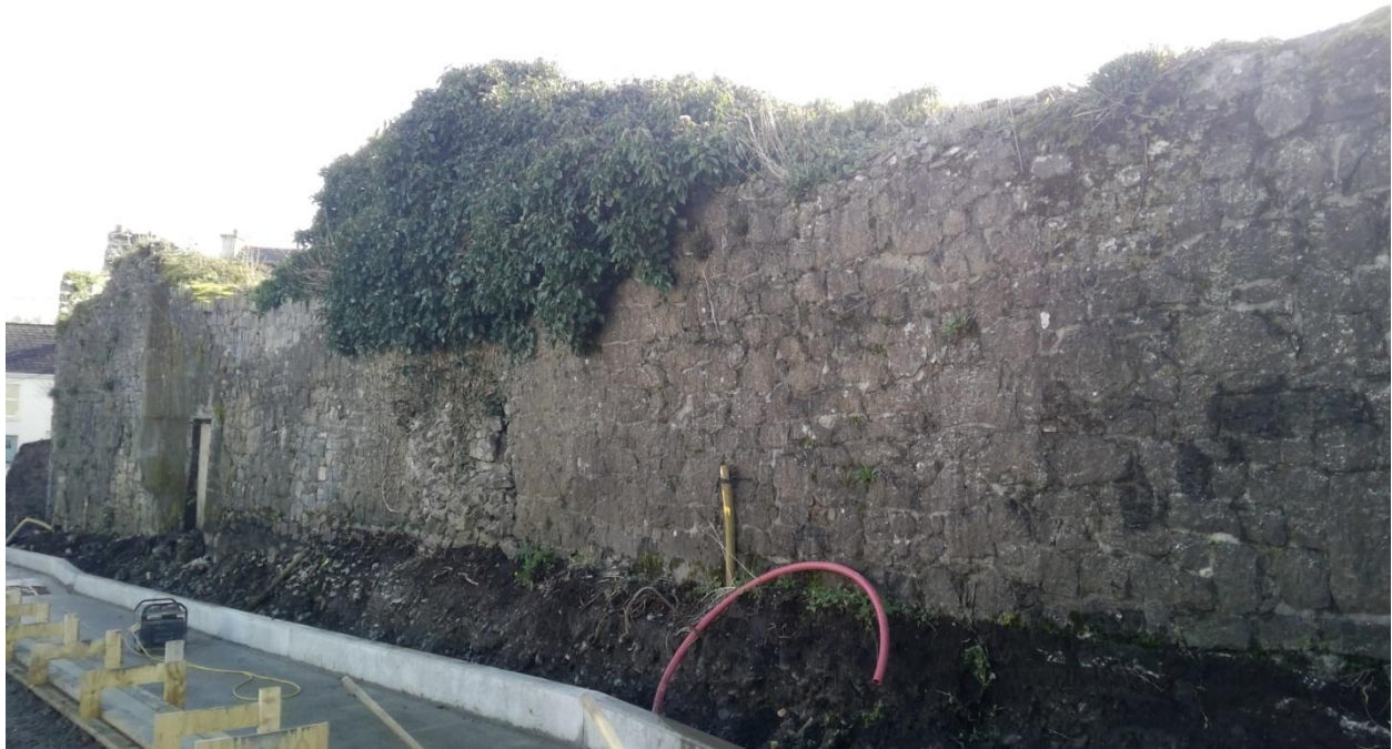
Pic 4: Significant ivy growth and vegetation on upper part of wall. This vegetation threatens the fabric of the wall and is to be removed in tandem with the re-pointing and consolidation of the wall.
