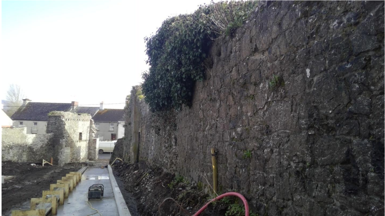
Pic 6: General view showing the presentation of the town wall within the new park. The upper part of the wall has been colonised by heavy ivy growth, which has broken down the haunch and threatens the stability of the wall.
