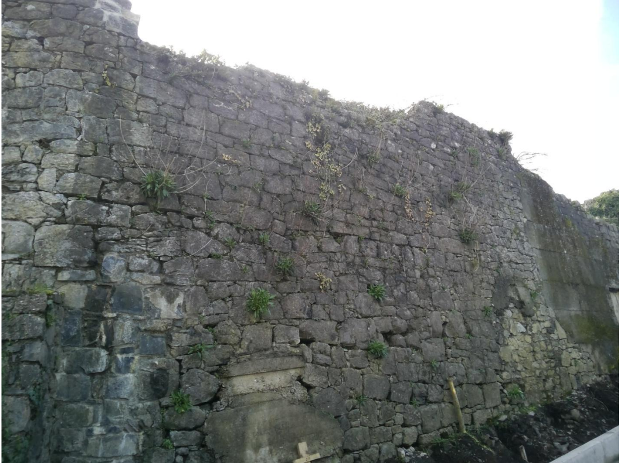
Pic 2: This photograph shows the southern part of the subject wall (northeast face), viewed from within the new park. There are areas of missing mortar, together with gaps and cavities associated with missing stones.
