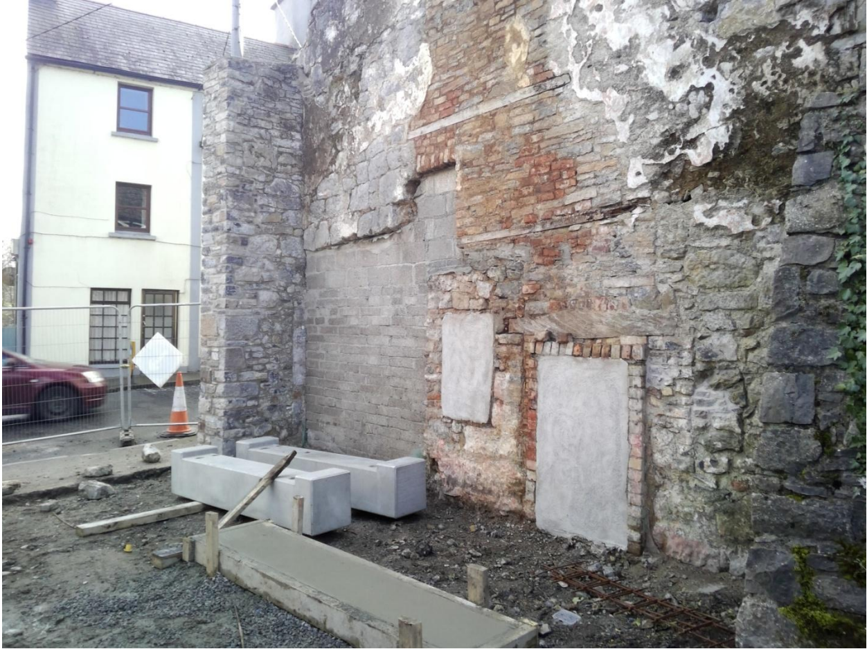
Pic 9: Section of wall at entrance to new park from Burke St., with blockwork infill panel to be finished with a lime harling.
