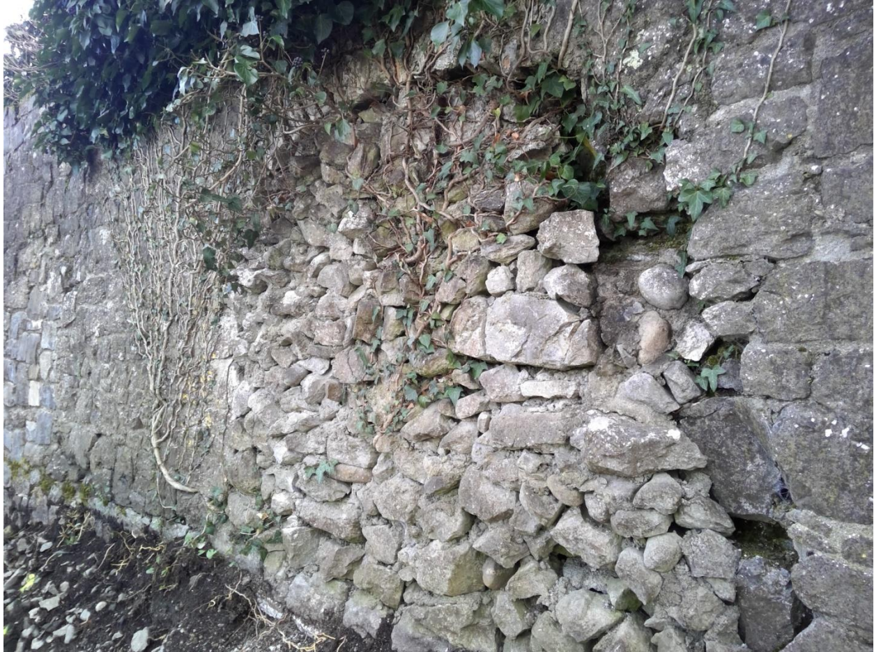
Pic 5: Location of earlier opening within the wall. The infill rubble within the wall was presented as a rougher finish than the dressed rubble of the main wall, during previous works carried out in 2009. There has been a loss of mortar and colonisation of the open joints with ivy within this infill masonry. The dressed stone, around the perimeter of the opening required consolidation.
